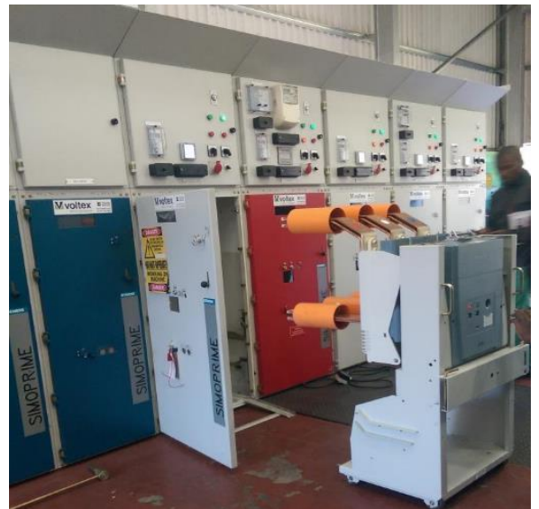
MEDIUM VOLTAGE SWITCHING (11 000 VOLT)
