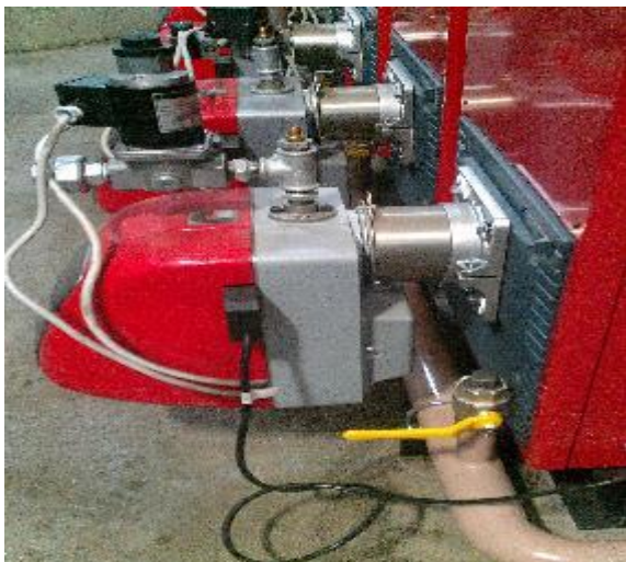
Gas Burner incident
