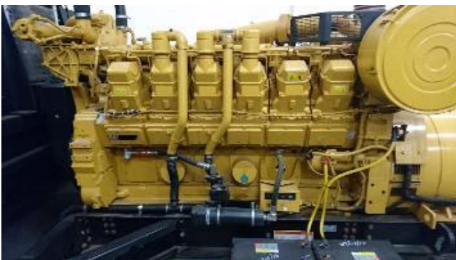
Standby Generator engine and electrical maintenance
